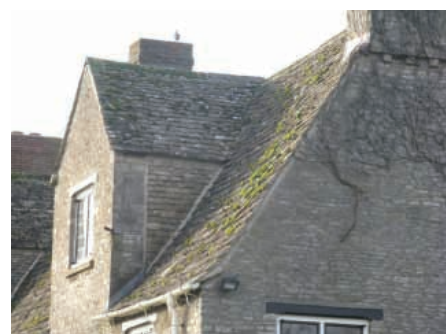
Repairs using traditional materials add to the aesthetic appearance of a property, as the new stone slates on the dormer at no. 42 show
